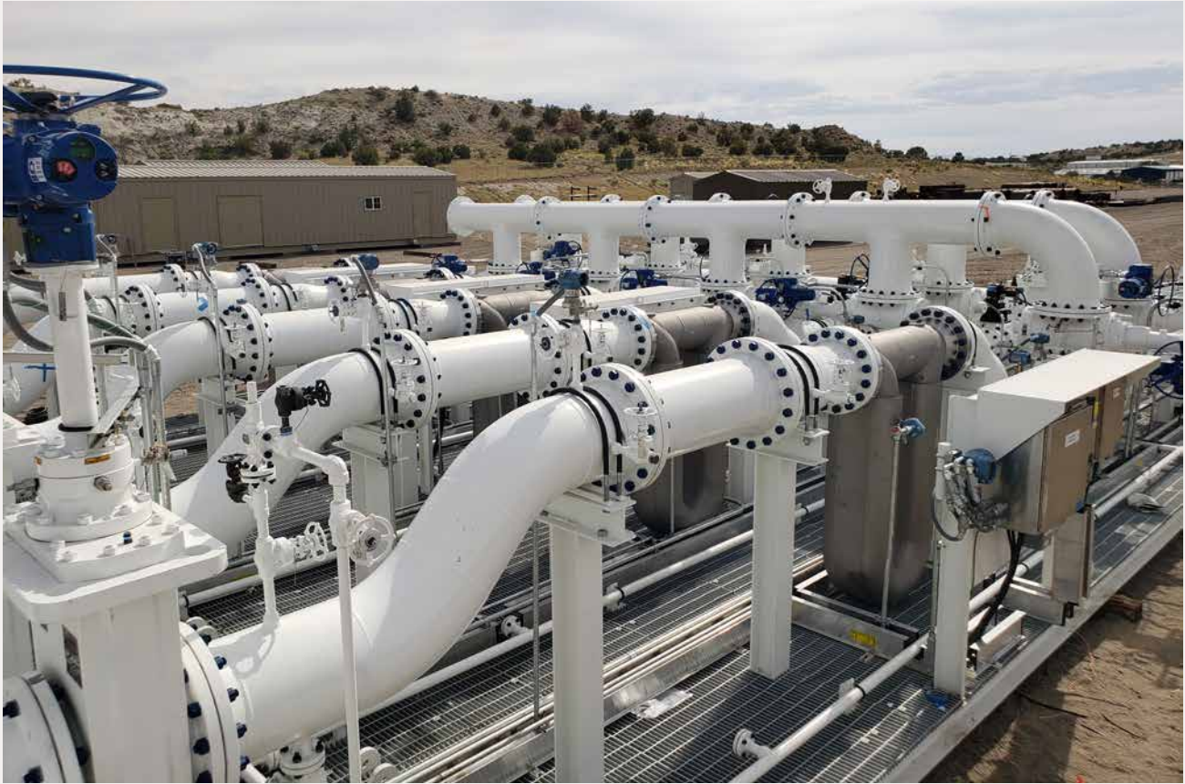
Crude Oil Pipeline Metering Skid
